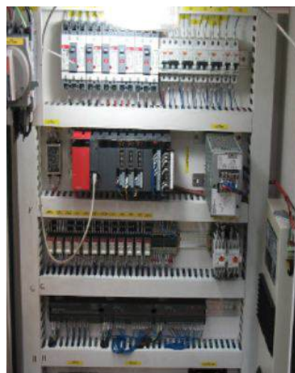
Main Control Panel
