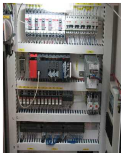
Main Control Panel
